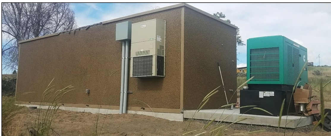
Example Regeneration Hut Housing an In-Line Amplifier
