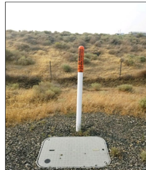
Typical Vault and Line Marker
